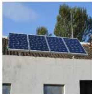
Figure 6. Solar panels installed.
