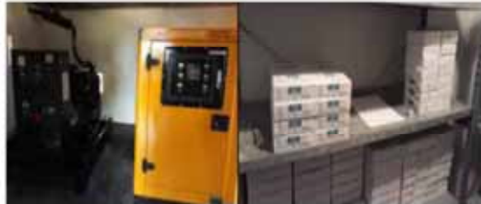
Left to right: generator; cold room Source: Mission team
